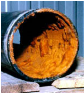
* Sample of sprinkler piping with obstruction
